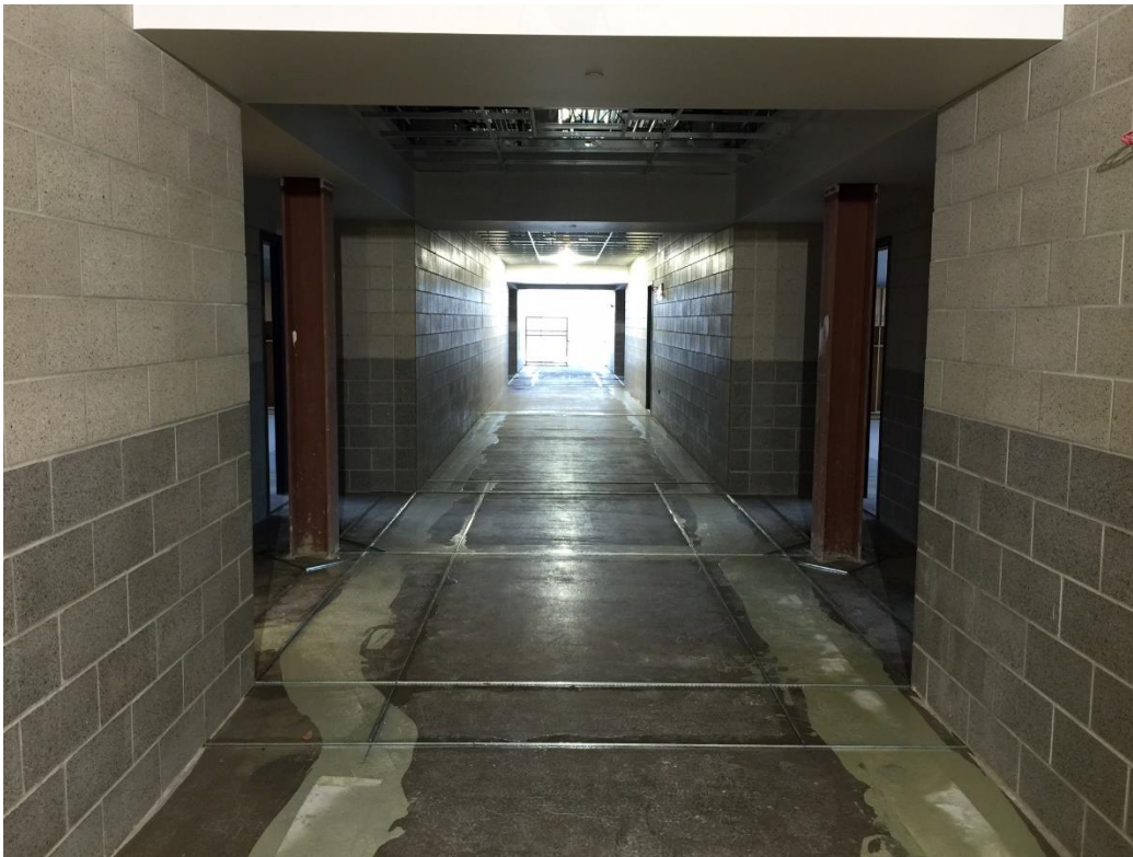
Terrazzo metal joints
