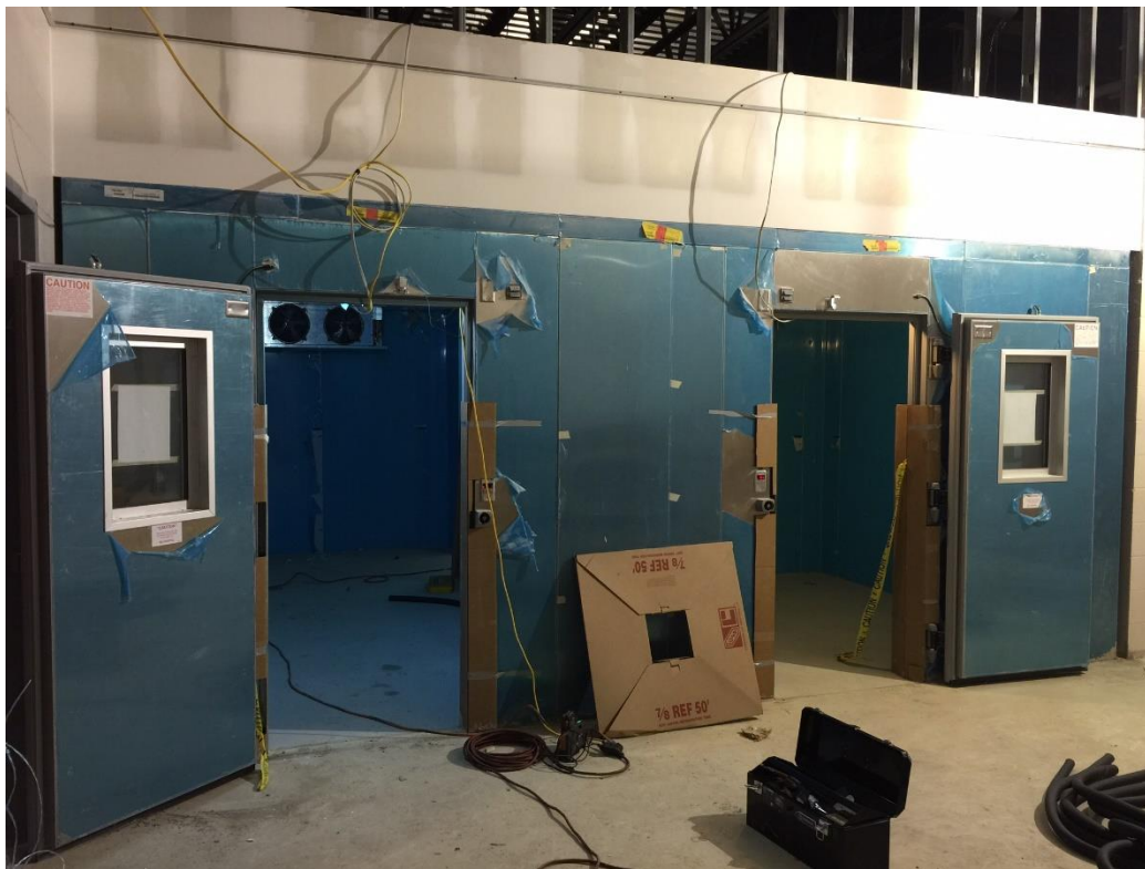
Freezer and cooler
